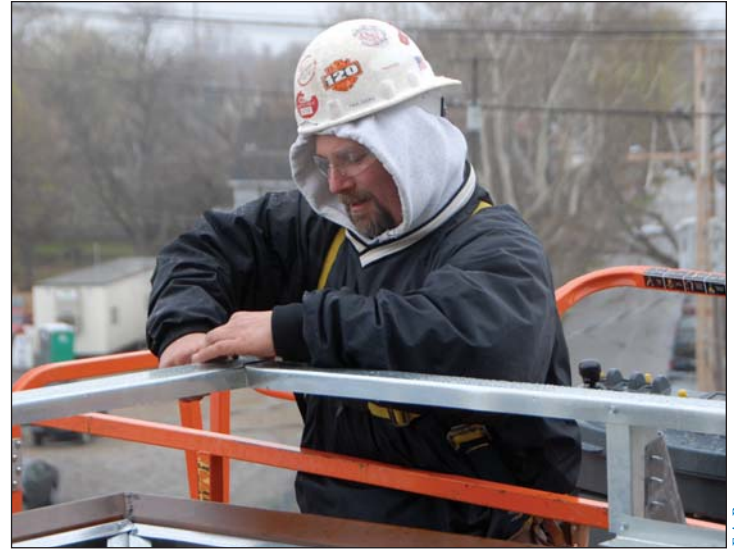
Carpenter "Chicken Joe" Corrin installs framing for cornice on the Juvenile Justice Center Project.
