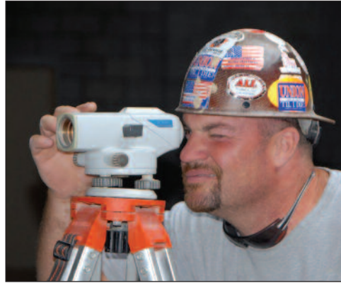
Chad Wienhold, brick mason, operates the transit level gun to shoot heights for block walls
